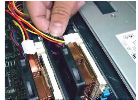
Connecting the power cable to the first PL-P3/SMP.
